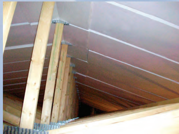
Custom cut eps-lite used to insulate an attic, including the tailored nook for the peak.
