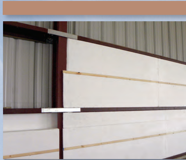
Customized eps-lite used to insulate a machine shed with two layers of foam to eliminate common seams, with the outer layer including an accessible furring strip.
