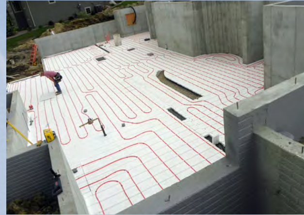
Thermo-Snap™ proved to be a worthy fit for this residential project that required several cutouts and a distinctive perimeter.
