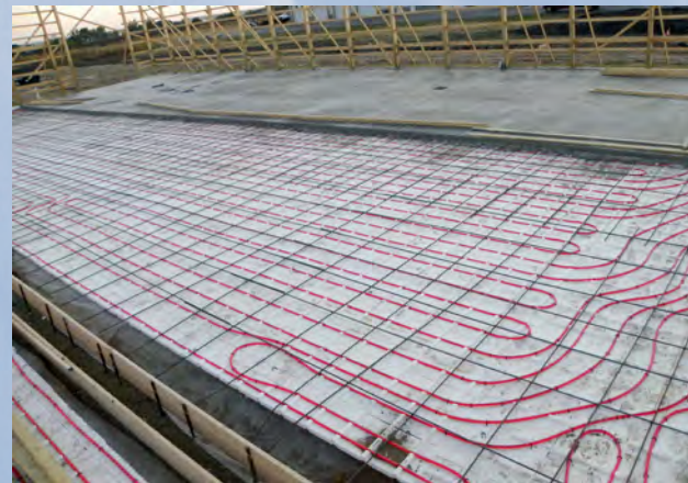
Installers at this commercial truck shop appreciated the quick and easy application of Thermo-Snap™ for this 7,000-sq-ft building.
